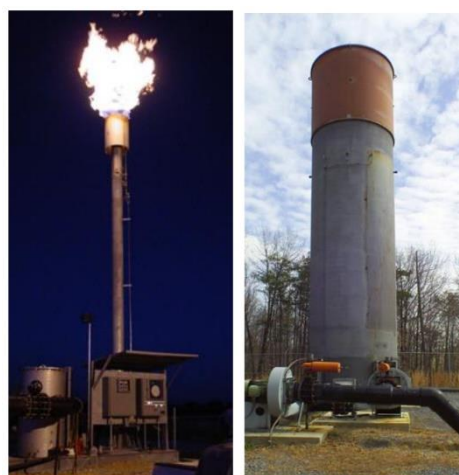
Figure 17: Open flare (left) and enclosed flare (right) (GMI 2012)
